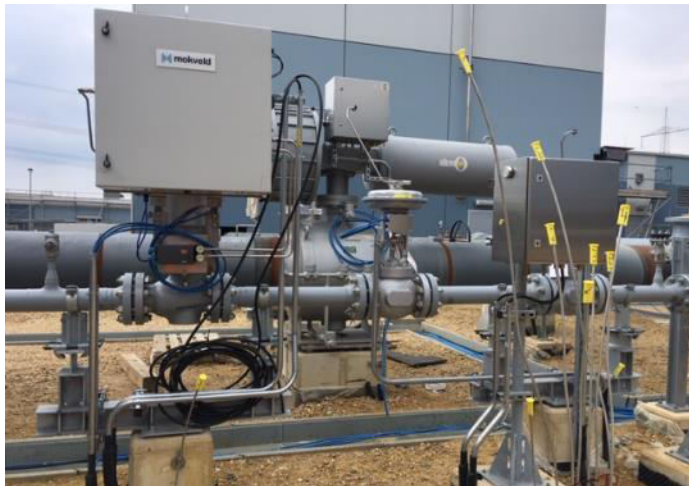
PROCESS AREA – ACTUATED VALVES
