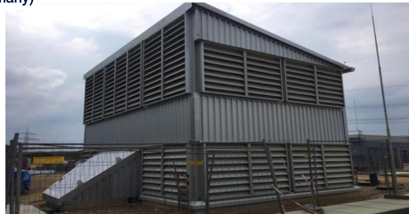
STEP UP TRANSFORMER AND SHELTER
