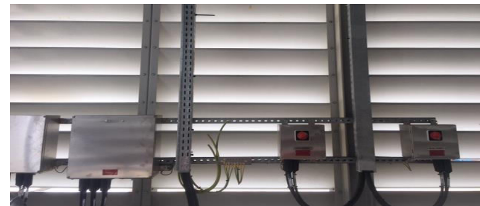
JUNCTION BOX CONNECTION AND SUPPLY
