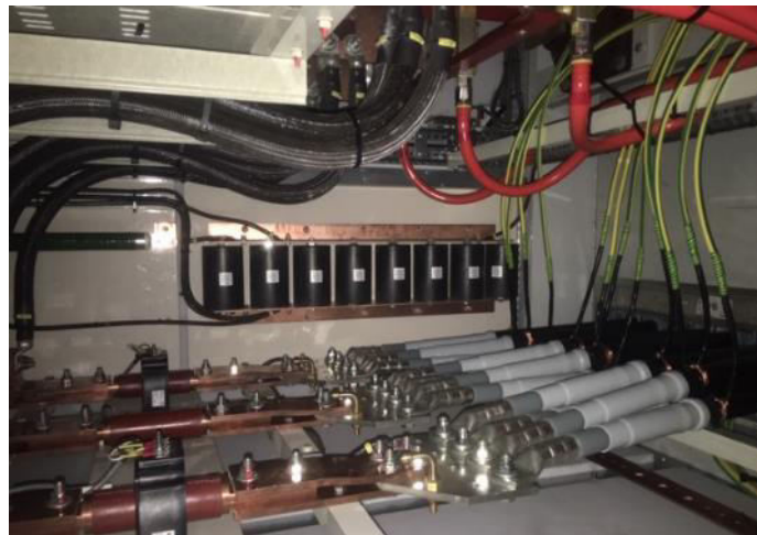
MV CABLES CONNECTION ON VFD PANELS
