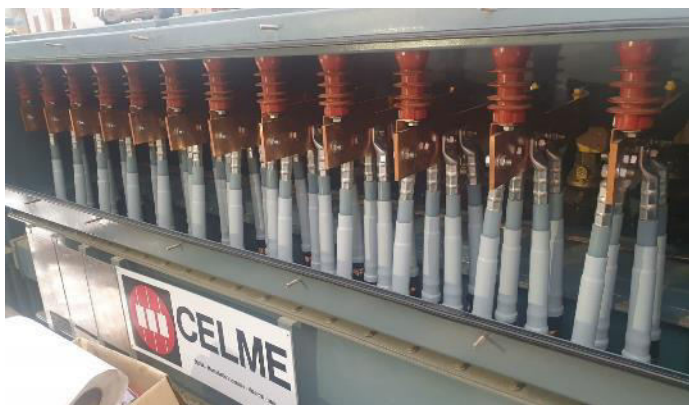
MV CABLES CONNECTION ON TRAF0
